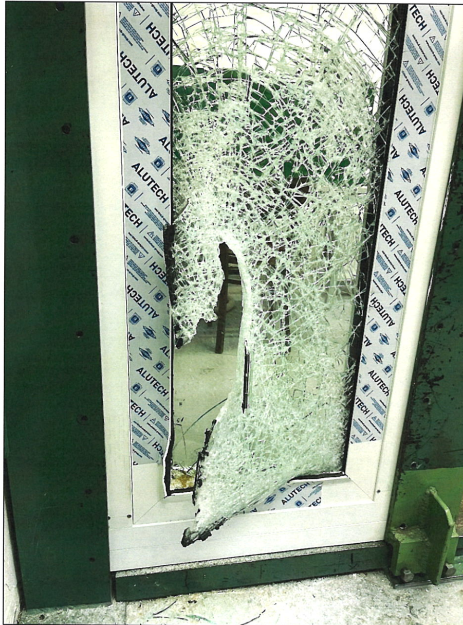
Pic. 16 – test sample No. 12/2023-3 after manual test No. 7 (view from the side of the attack – outside)
